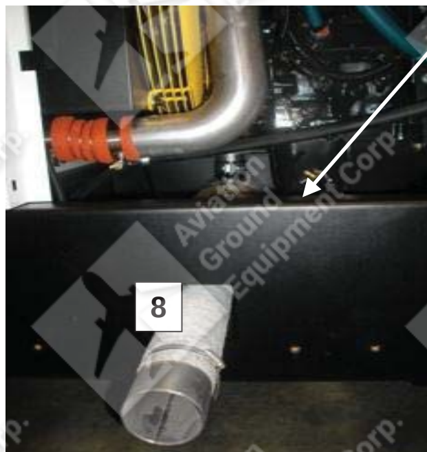
Figure 13 Engine Exhaust Components
